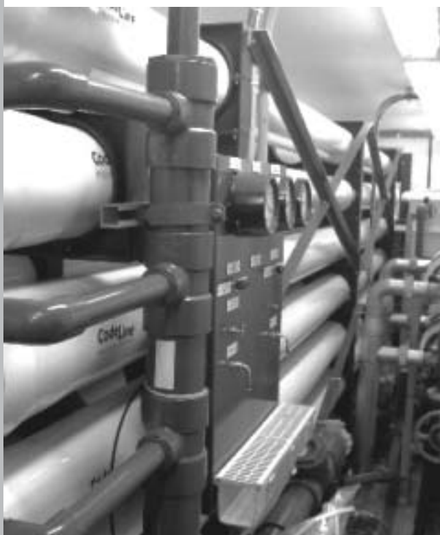
RO Plant at TCL-Mithapur
