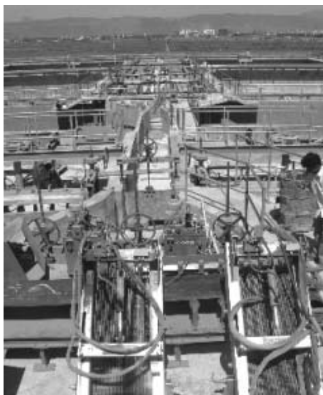
STP Plant at Jaipur
