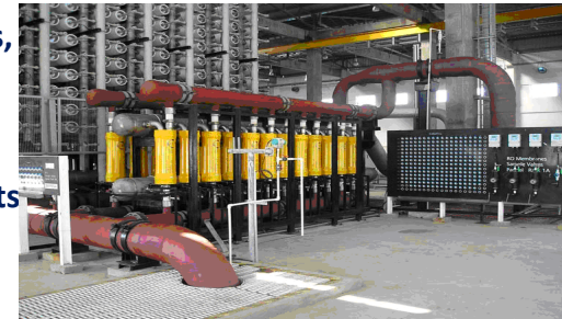
100 MLD Chennai Desalination Plant for Chennai Metro Water Supply
