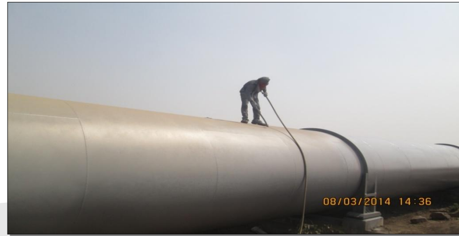
Tansa Transmission Main Pipeline, Maharashtra
