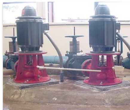
Vertical Turbine Pumps: 298 Highest Capacity 19.50 MW
