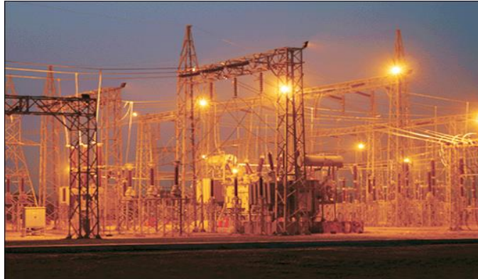
220/132KV Substations at ahadurgarh Haryana
