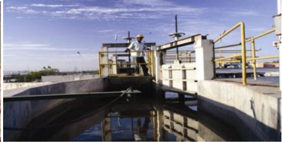
Sewage Pumping Station at Chennai
