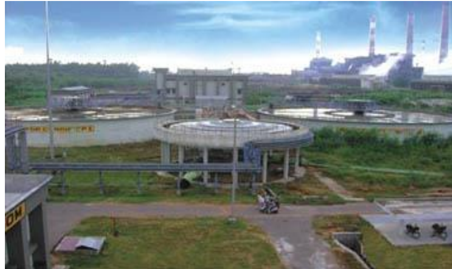
Vindhyachal Super Thermal Power Project NTPC-2X500MW Pre Water Treatment Plant
