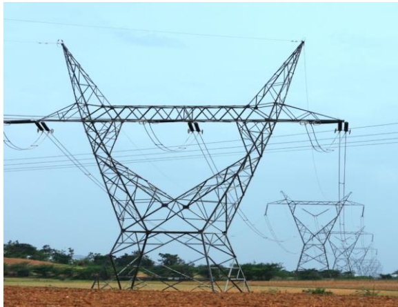
1,460 km of Transmission Lines (132, 220, 400, 765 KV)
