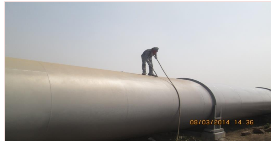
Tansa Transmission Main Pipeline, Maharashtra
